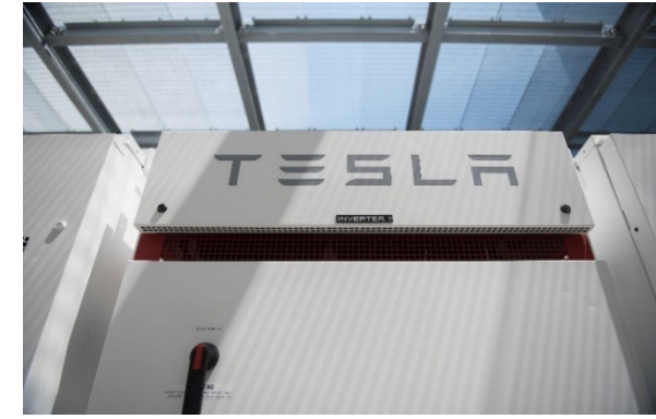
Battery Energy Storage Systems
