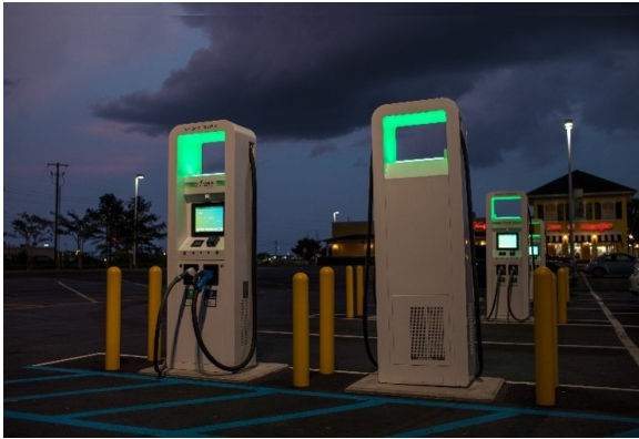
Electric Vehicle Charging
